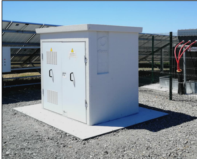
Plate 3-9. Outdoor cabin switchgear
