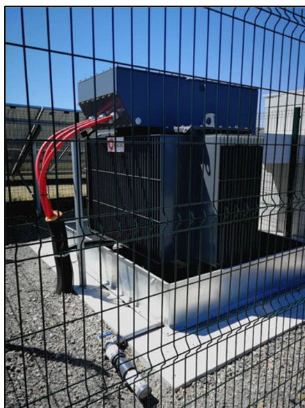
Plate 3-8. Typical outdoor transformer
