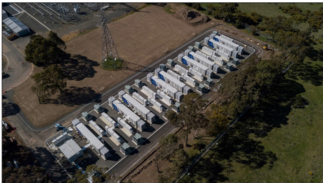
Plate 3-11. Typical battery storage compound configuration (image reproduced courtesy of Fluence Energy).
