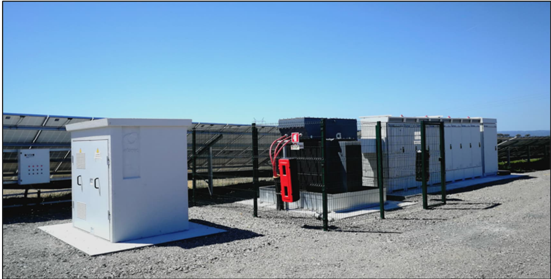
Plate 3-4. Outdoor solar station
