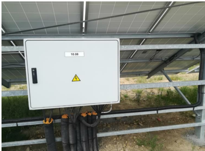
Plate 3-2. DC Electrical Box
