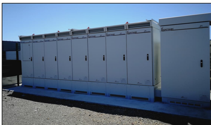
Plate 3-7. Typical outdoor centralised inverter
